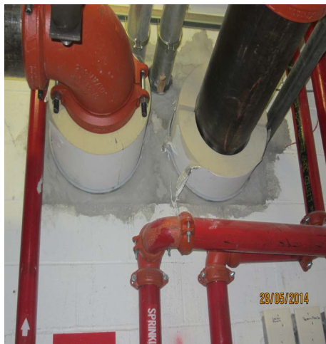
Sprinkler room firestop.
